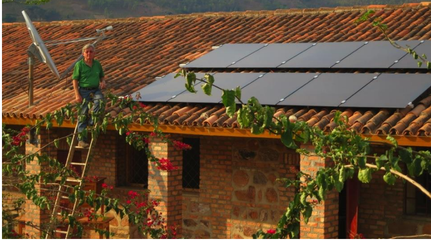
Satellite antenna e fotovoltaic panels
